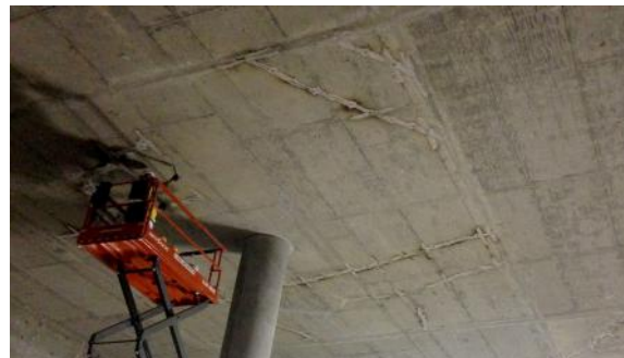
Repair of full-depth shrinkage cracking on the underside of the roof deck.
