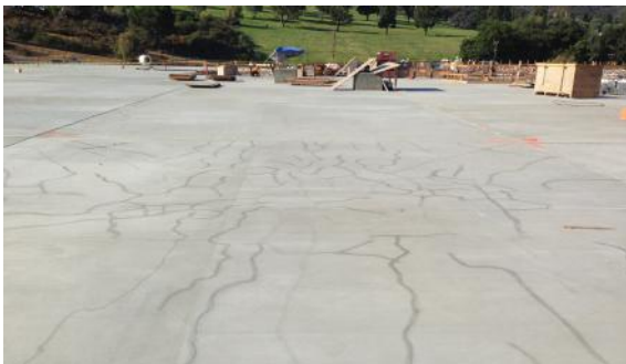
Typical roof deck shrinkage cracking (without the use of PREVENT-C).
