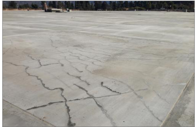
Typical roof deck slab showing extensive full-depth shrinkage cracks. These cracks are shown after epoxy injection repair and skim coating. Other minor cracking occurred but is not visible.
